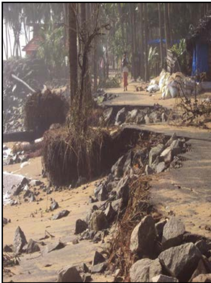
Fig. 7: Damaged road at Vadanapilly coast
